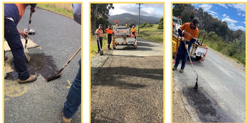
Above: Recent Emulsion Spraying Works on Saltwater River Road, Blowhole Road and Safety Cove Road
